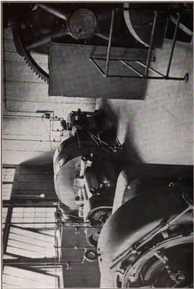
PLATE 6.—STOP ARRANGEMENT OVER ROLLING MACHINES By pulling the rope which the operator is holding, the switch is thrown out and the motor driving machinery is instantly stopped
